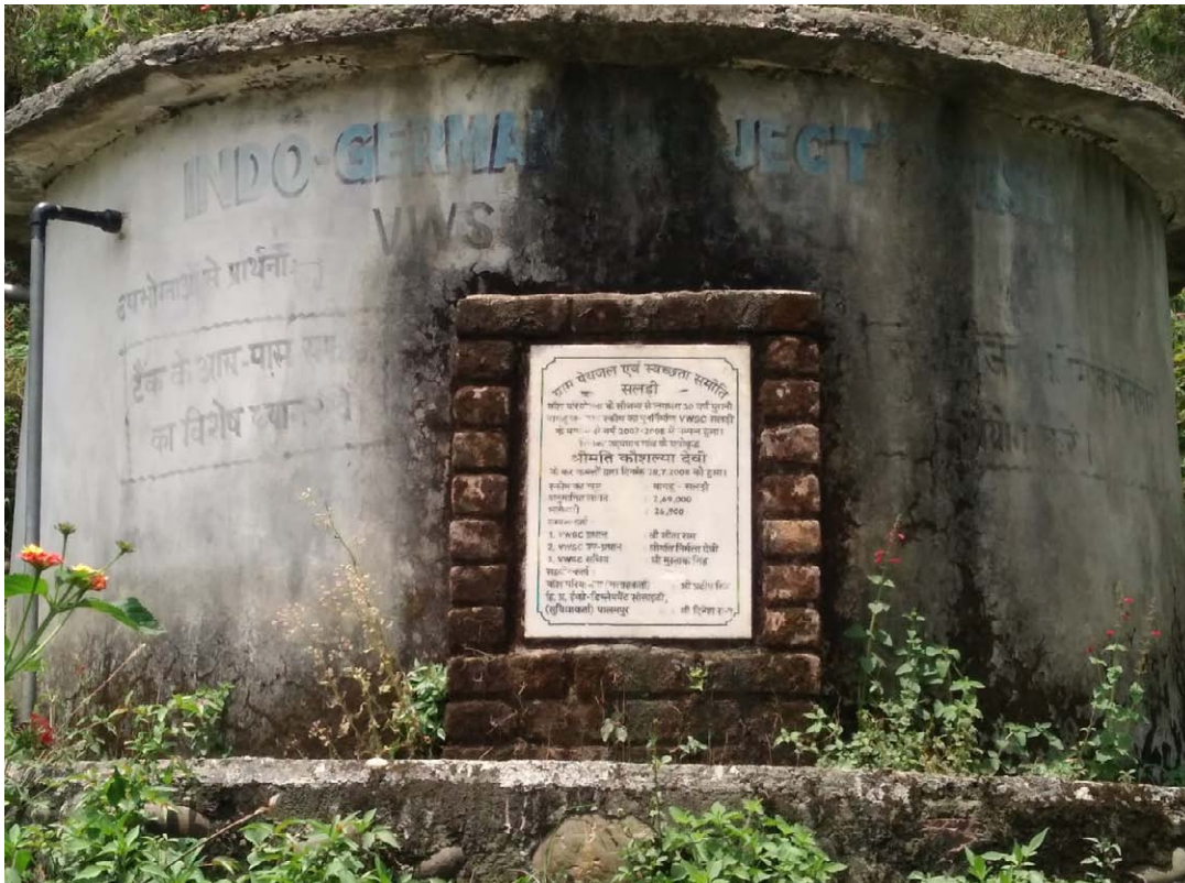
Example of a community water tank installed during the Indo-German Changar Eco-Development Project (India). Such water storage structures proved successful in improving community well-being in regions affected by water scarcity. © S. Srigiri
