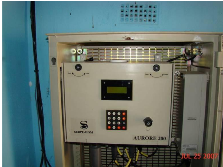
Figure A4.2: A typical AURORE logging unit with the transmitter on the right hand side.
