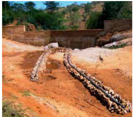
An infiltration gallery connected to an external tap, installed during construction.
